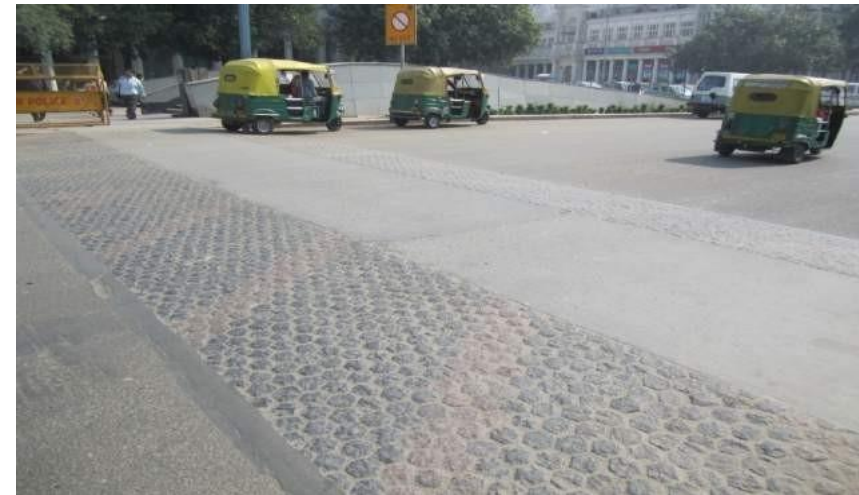
Photo 5.3 Tabletop with cobble stone on slope and cement concrete surface on top
